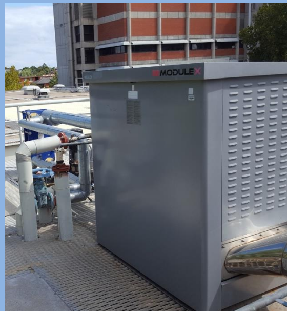
Gas Boiler and Its Primary Pump
