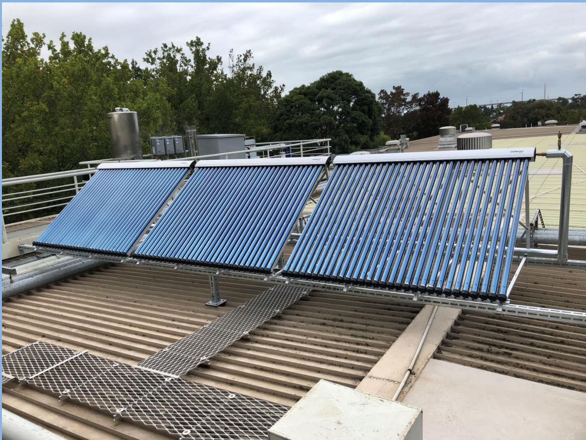
New Solar Hot Water System with Gas Boosters
